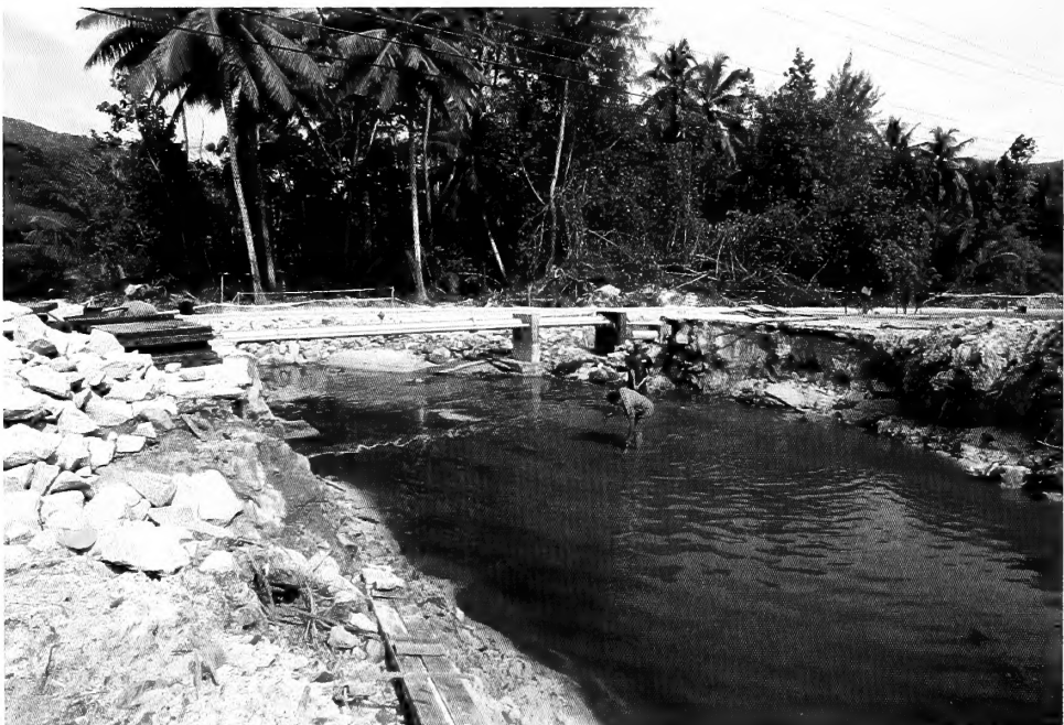
Plate 4. Road bridge washout following drainage of tsunami waters, southwest Mahé.
