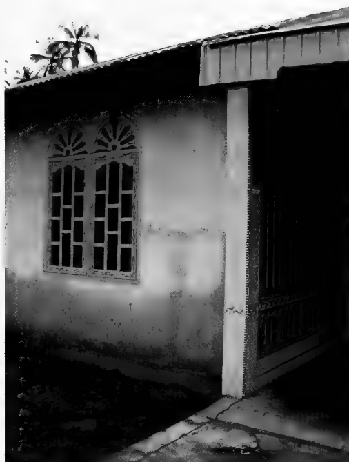
Figure 5. Water mark on house on Pulau Baleh; mark represents the daily height of water inundation at high tide. This house is approximately 70 m inland.
