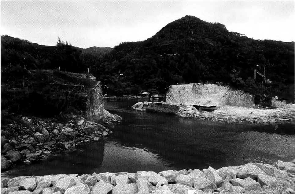
Plate 3. Road bridge washout from seaward drainage of tsunami waters from coastal lagoon, west coast of Mahé.
