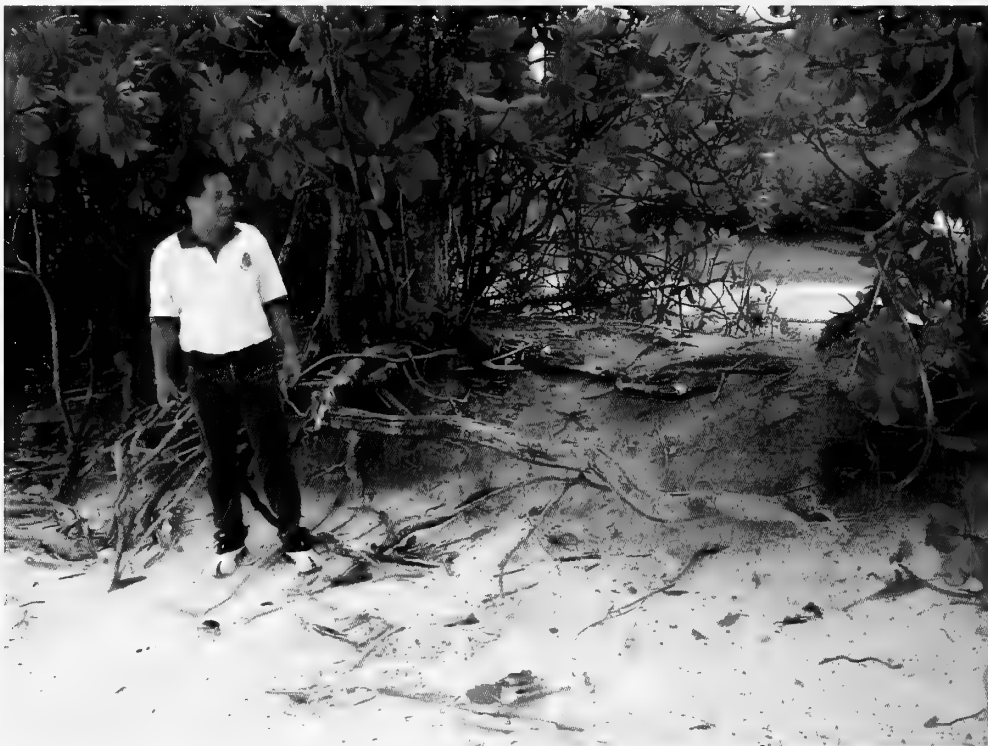
Figure 5. Erosion of the seaward side of the western arm of Diego Garcia. The observer is standing on the high tide level, the thin rim behind him is now all that stops inundation of the road at this point.
