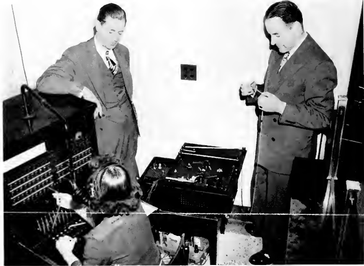
Edith Hingley, KDKA-Pittsburgh switchboard operator listens while T. C. Kenney, Chief Engineer, and J. E. Baudino, General Manager, explain the technical phases of the station's telephone answering gimmick. A magnetic tape recorder specially rigged to the outlet's switchboard played back recorded "hellos" of network stars to incoming callers—KDKA's way of hyping listener interest in web shows.
