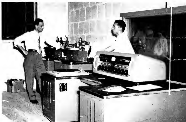
Disc recorders and control console being installed in Protestant Radio Center's headquarters, at Music Building of Agness Scott College, Decatur, Georgia.
