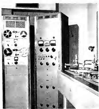
The "business end" of WMBI's sound recording room, showing rack mounted Magnecorder tape machines, audio amplifier equipment and two Presto disc recorders.
