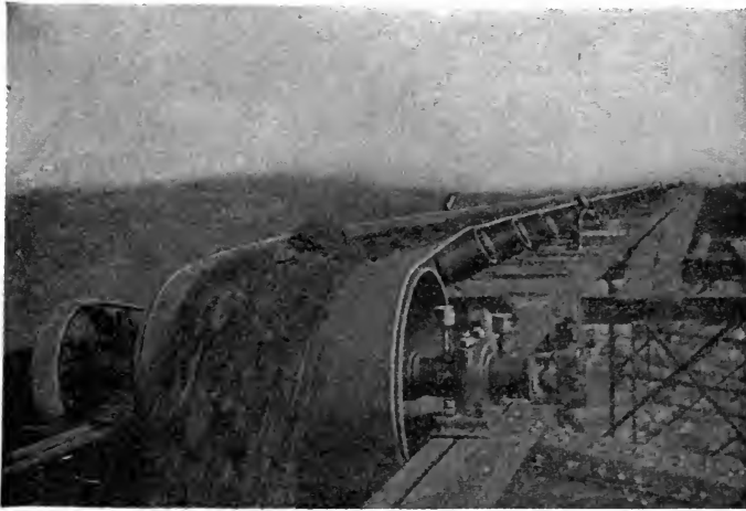
FIG. 314.—Discharge at Head of Conveyor.
