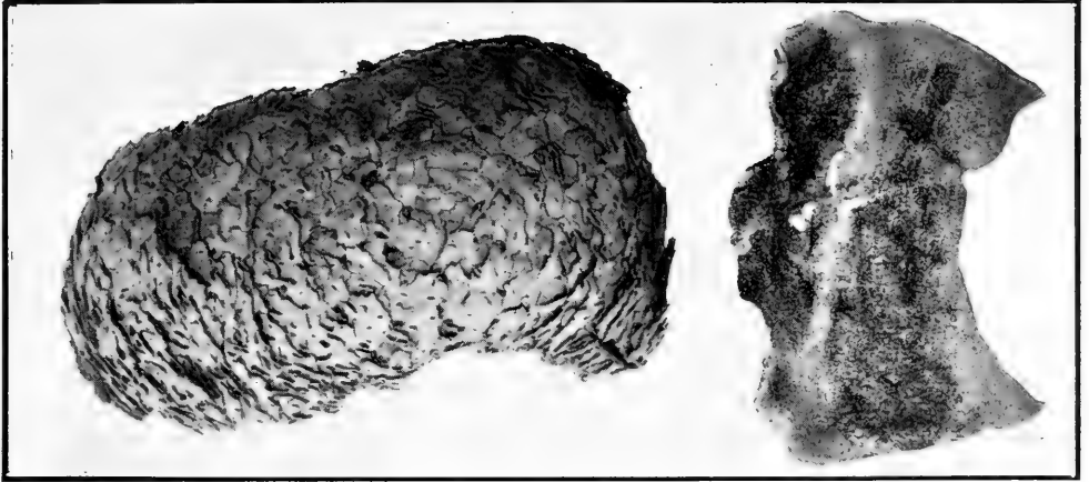
The lead was eaten through by “White Ants” so that they could attack the wood in the roof of the Museum. The nest shown on the left was removed from a beam in 1896.
