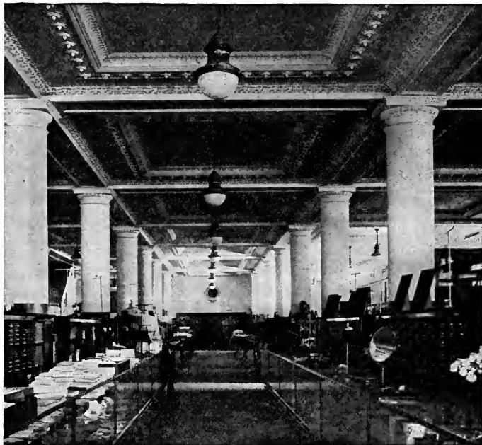
GRINNELL SPRINKLERS IN A DEPARTMENT STORE. PIPING CONCEALED AND CEILING DECORATED BY ROSETTES OF A SIMILAR SHAPE TO A SPRINKLER. ROSETTES OMITTED AT PROPER PLACES AND SPRINKLERS SUBSTITUTED.
