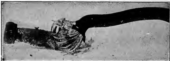
FIG. 64.—Effect of corrosion on battery cable terminals.
