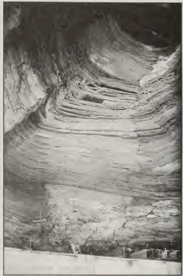
Figure 35 Large roof fall in laminated Energy Shale, Jefferson County (Coal Section files, ISGS).
