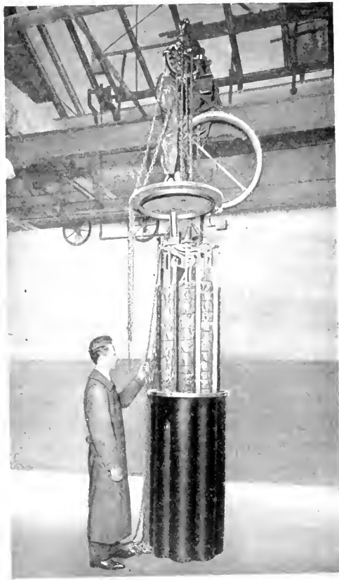
Fig. 17—Assembly of 300-coil case Lowering loading coils into case after coil spindles have been mounted on frame and coil terminals spliced to stub cable conductors
