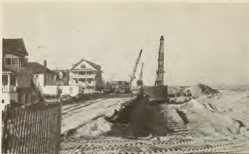
Figure 11. Sea Isle City bulkhead under construction just north of profile line 14, April 1963.
