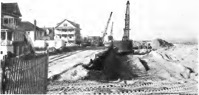
Figure 11. Sea Isle City bulkhead under construction just north of profile line 14, April 1963.
