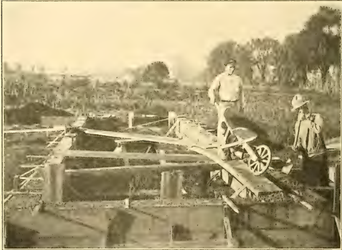
At Work on Solid Concrete Foundation, New Jersey Experiment Station. Note Removable Forms and Binding Braces
