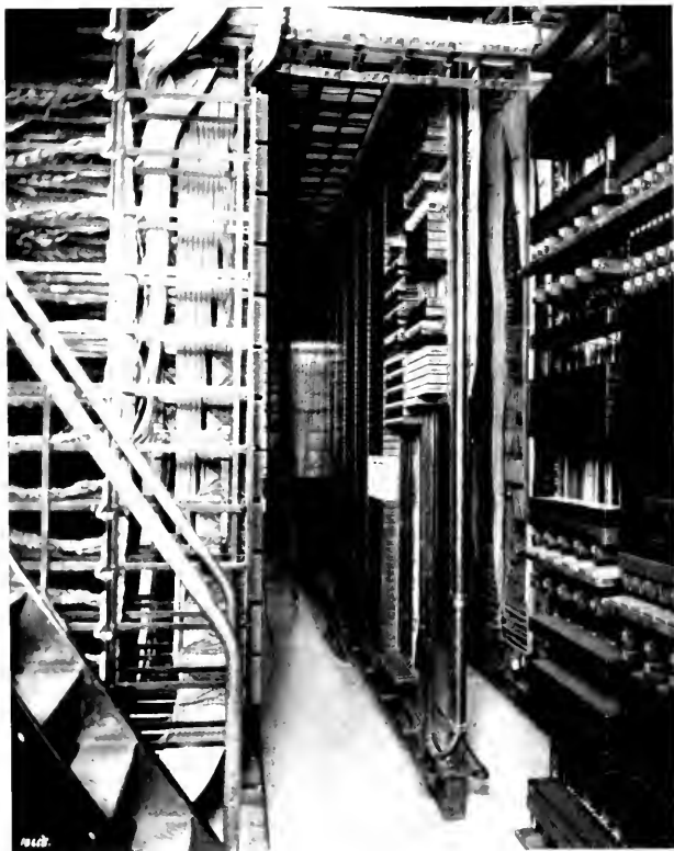
Fig. 1—Relays in a local manual office
