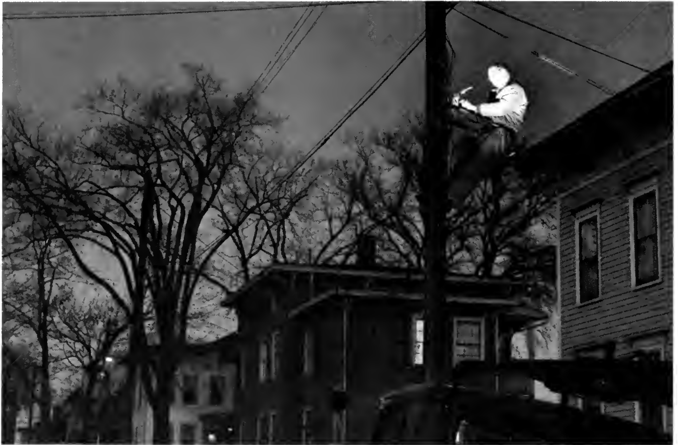
"If it's an emergency to you, it's an emergency to us"—a Southern New England Telephone Company repairman restores service to a
