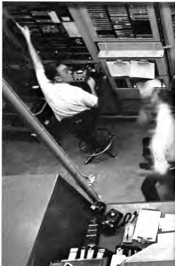
Central office repairmen in Richmond man the test board of a $10 million switching machine. Such large plant investments are essential to fulfill modern communications needs.
