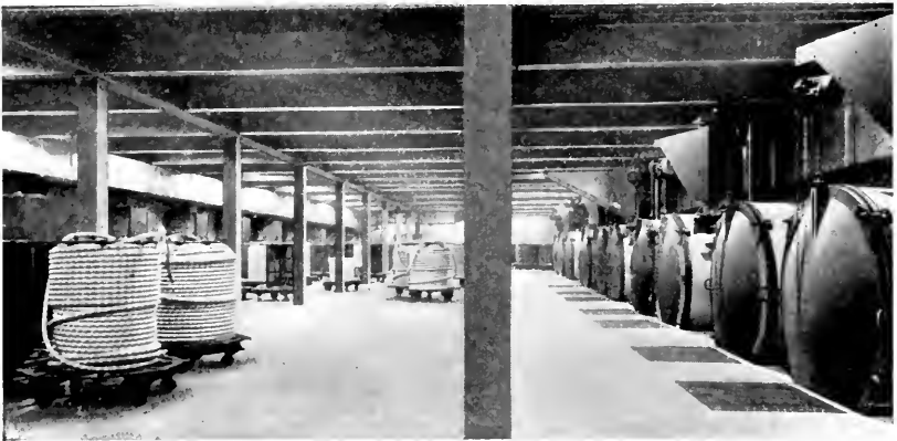
Fig. 17—Air conditioned cable storage room.
