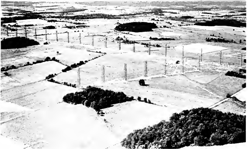
Fig. 5—Lawrenceville transmitting station. Aerial view—South American antenna in the foreground; European antenna in the background. Two buildings each containing two transmitters are shown.
