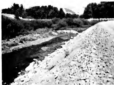
A section of Flint Creek after adjacent highway construction.
