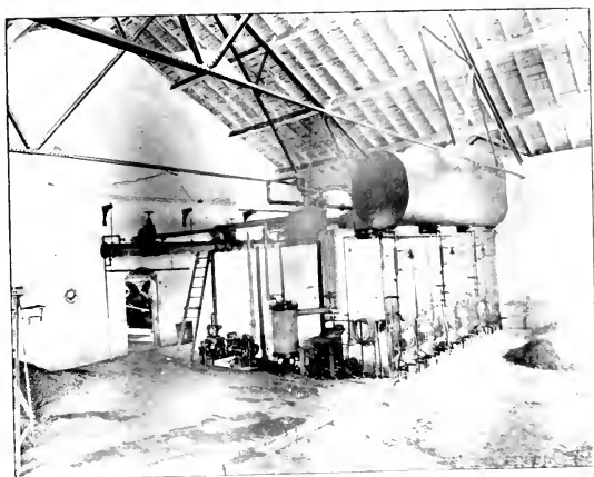
BOILER ROOM BINGHAMTON ELECTRIC RAILROAD.
