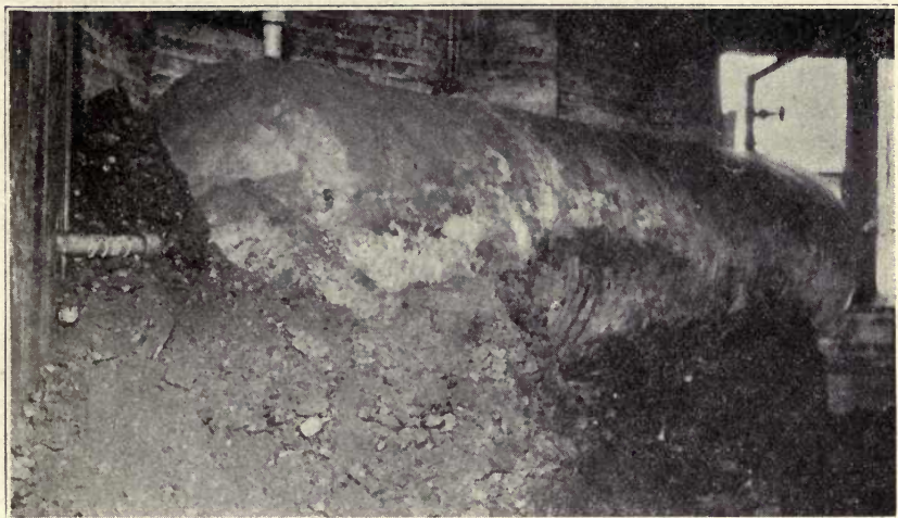
FIG. 16. COAL PILED AROUND HOT WATER TANK
