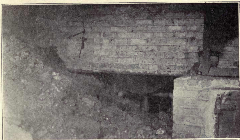
FIG. 20. COAL PILED IN CONTACT WITH BRICK WALL OF FURNACE (COAL HAS BEEN PARTIALLY REMOVED)
