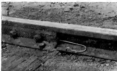
FIG. 2. BOND WIRE AT RAIL JOINT.
