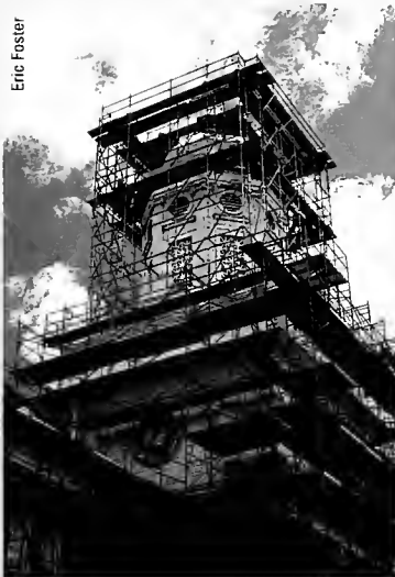
Carver Hall's tower and dome undergo substantial renovation during summer and fall 2002, with reinforcements installed inside and copper sheathing applied to the outside.
