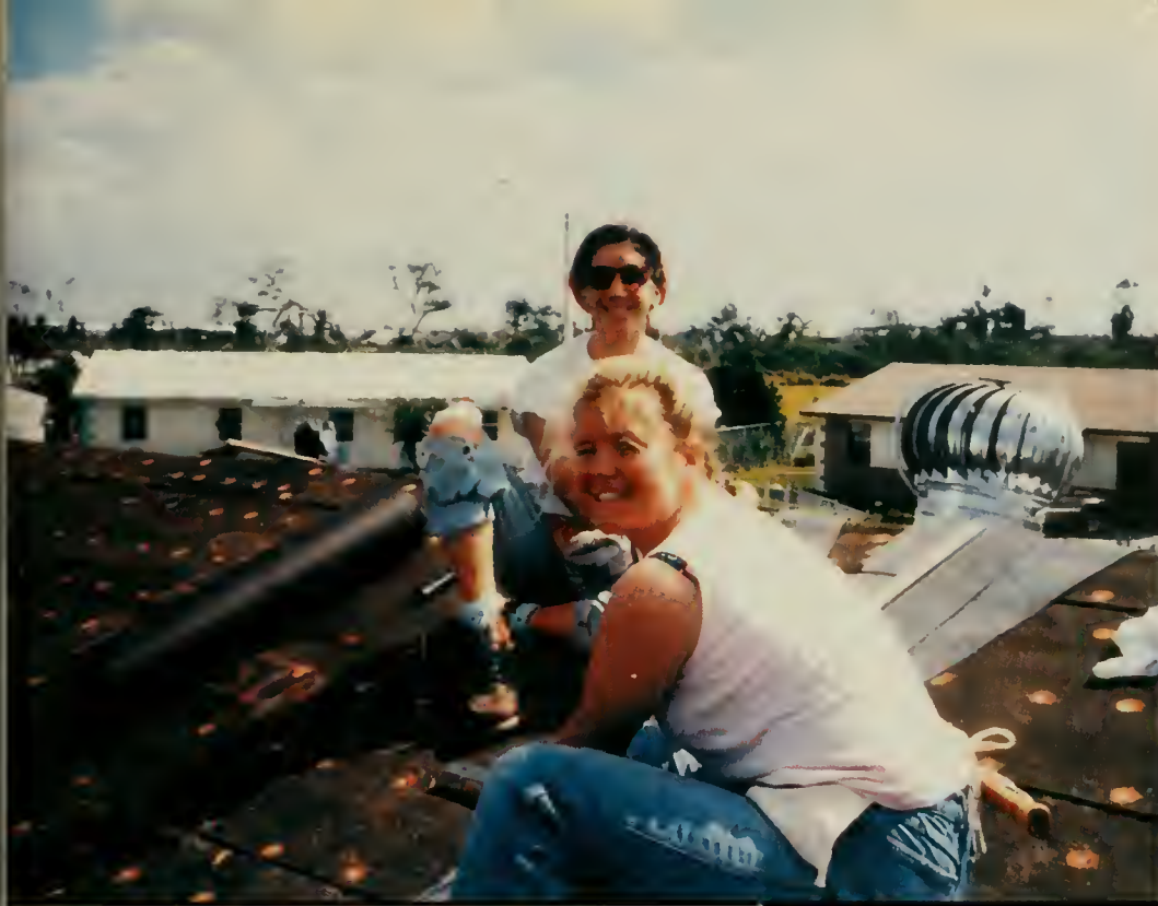
HAMMERING AWAY. Lauren Cogswell rebuilds one of the many roofs damaged by Hurricane Andrew. Several campus organizations sent relief groups to help for the week.
