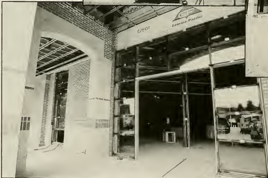
Transforming from a faculty parking lot in front of Godwin, to a brand new bookstore, the construction began in Spring 2002. The two story building was expected to be completed before the end of the fall semester. ■ Photos by Rachel O'Donnell and Jenny Brockwell
