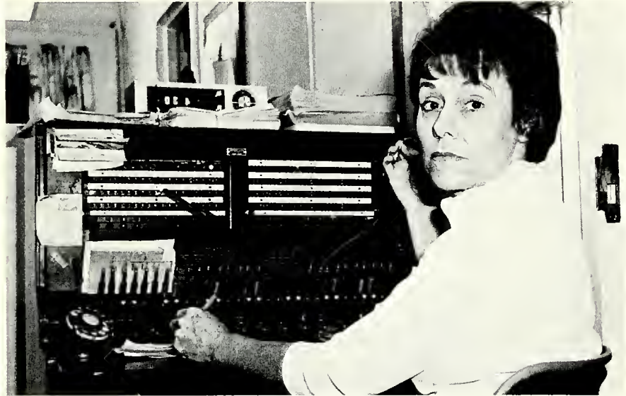
Virginia McCoy - Switchboard
