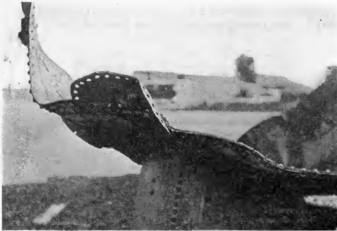
Fig. 3. Close-up view of patch and crack.
