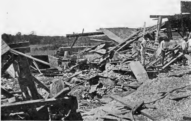
Fig. 1. Result of boiler explosion in planing mill, Antlers, Okla.
