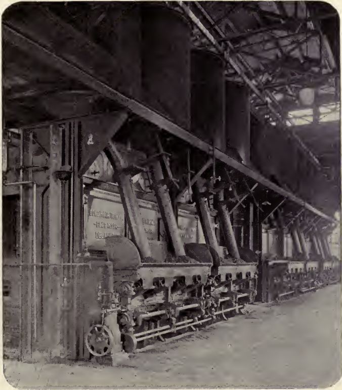
MONTROSE PUMPING STATION, ALLEGHENY, PA. Water-Tube Boilers.
