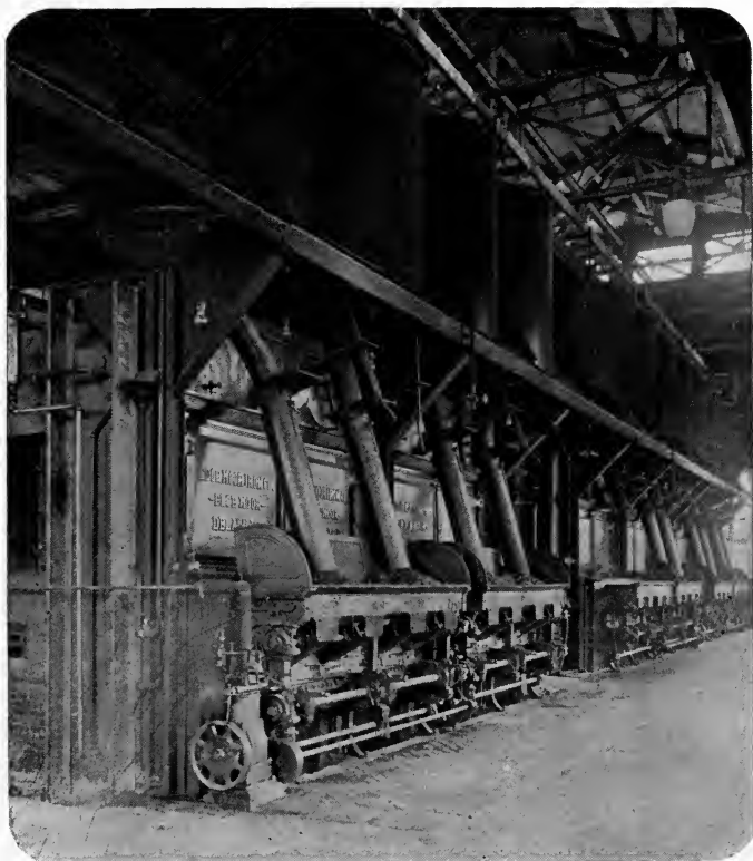
MONTROSE PUMPING STATION, ALLEGHENY, PA. Water-Tube Boilers.
