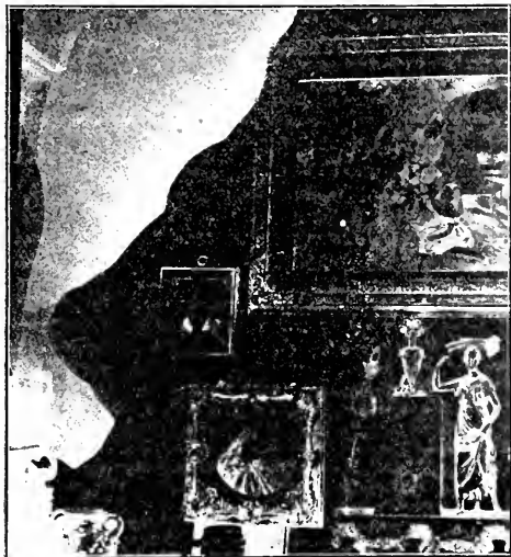
Fig. 213.—PATCHES DUE TO UNEVEN ACTION.
