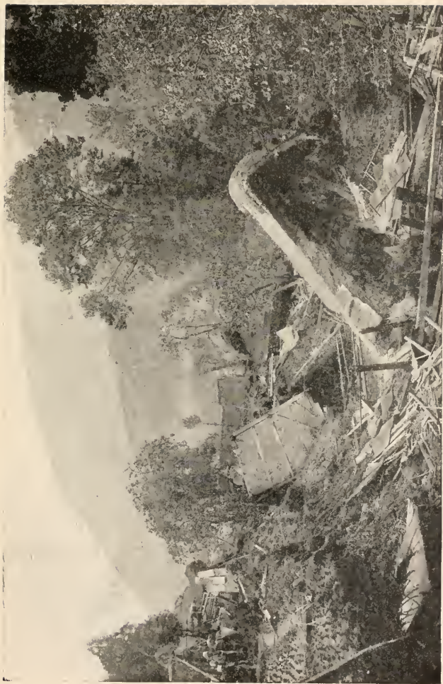
The Work of the Great Earthquake of 1891 in Neo Valley, Japan.
