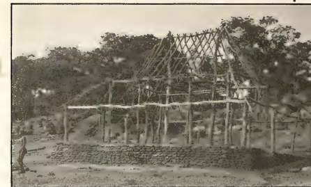
Above: A house under construction that was intended as a temporary home for the Hathaways. When completely finished the building was to be the workshop at Bassai.
