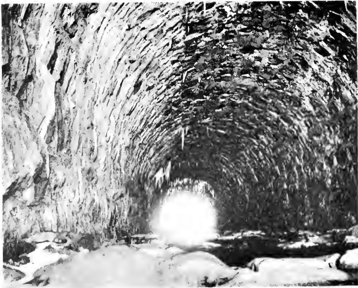
"CUSS GUTTER" CULVERT ICE EFFECT. Photo by F. W. Giddings.
