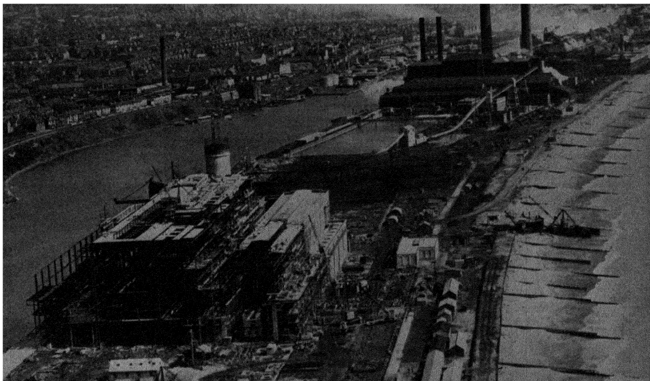
The Brighton "B" generating station (in foreground) under construction at Shoreham harbour, Sussex. The first half of the station was due to be completed in 1953. In the background is the existing Brighton generating station.
