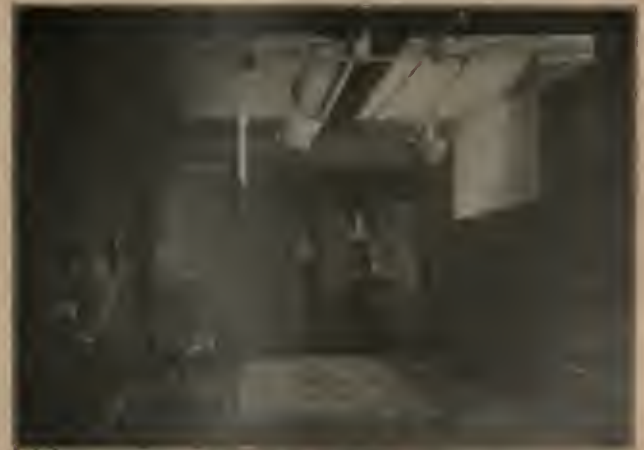
Fig. 1. Photograph of Mr. T. C. Turner's studio, showing adjustable reflectors mounted on rollers placed on each side of the half-watt installation and movable transversely.
