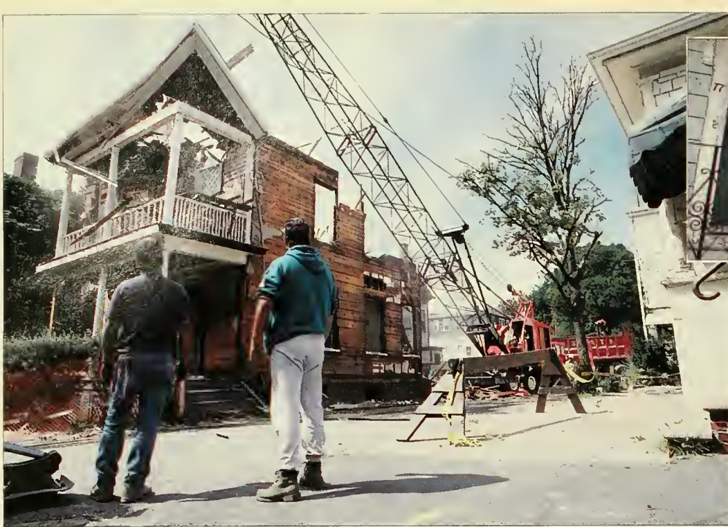
The walls of six dilapidated houses quickly came tumbling down on Brook Street (left) and Benevolent Street (above) after the city planning commission approved Brown's "master plan" for campus development.
