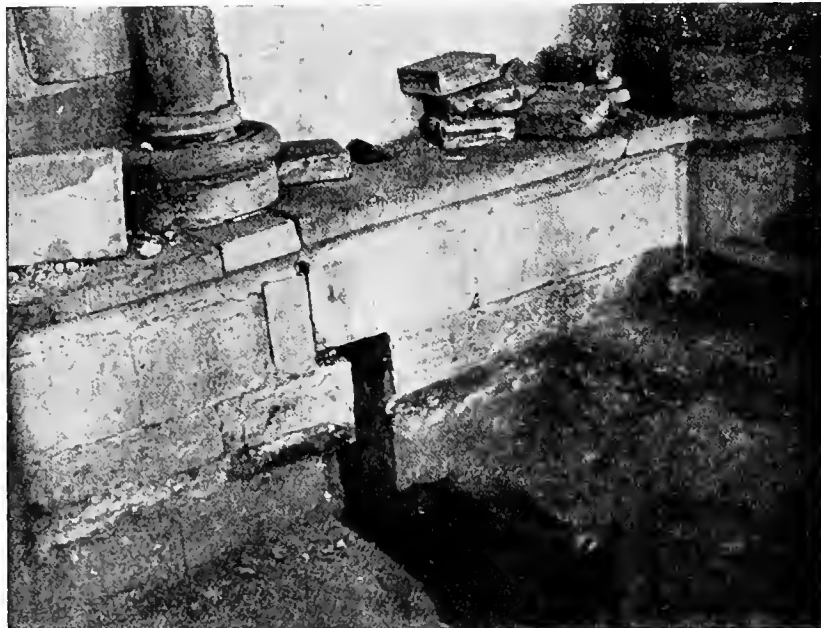
FISSURE IN FOUNDATIONS.
