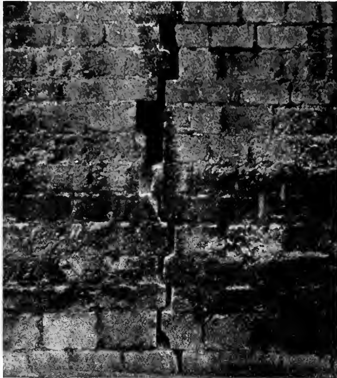
FISSURE IN NORTH TRANSEPT.
