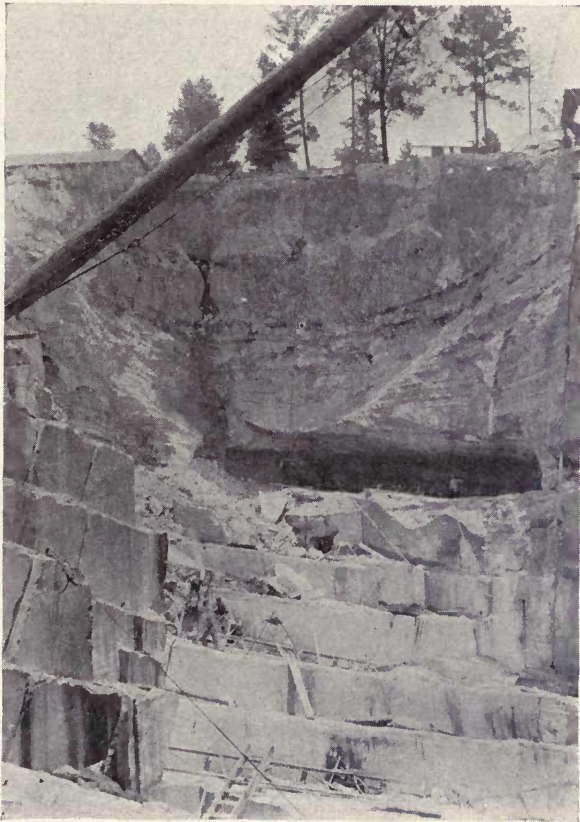
Fig. 137.—View showing the initial stages of a tunnel in a marble quarry in Alabama. Two tunnels are now utilized to increase the floor space of this quarry. Photo. by W. F. Prouty.
