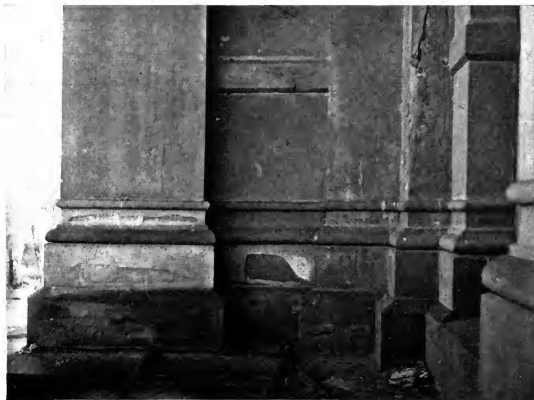
PLATE XVII, Fig. 2. — Weathered sandstone, second story, County Court House, Denver, Colo. (Photo by R. D. George.)
