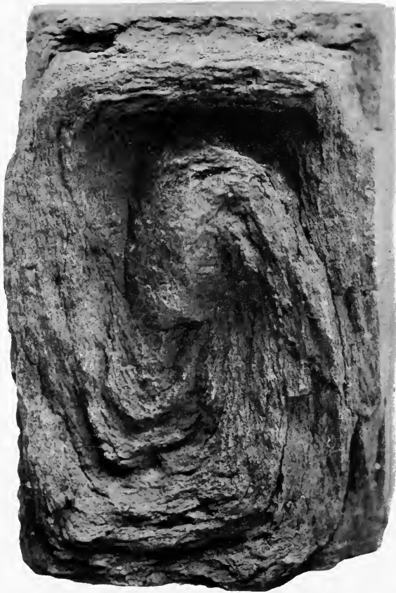
Plate XLVII. — Section of stiff-mud brick showing laminations.
