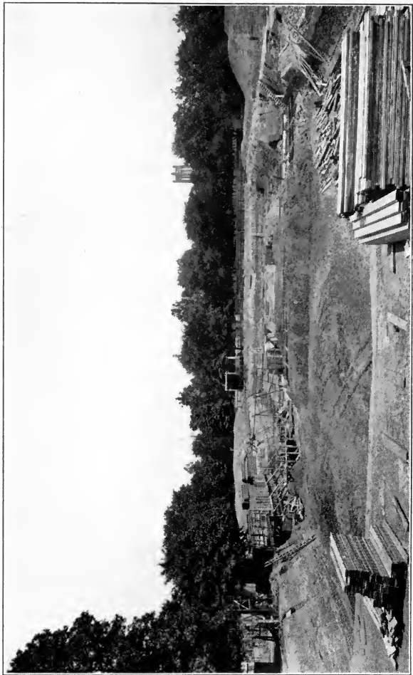
Excavating for foundation of new Art Museum. Appearance after two months' work, July 23, 1913
