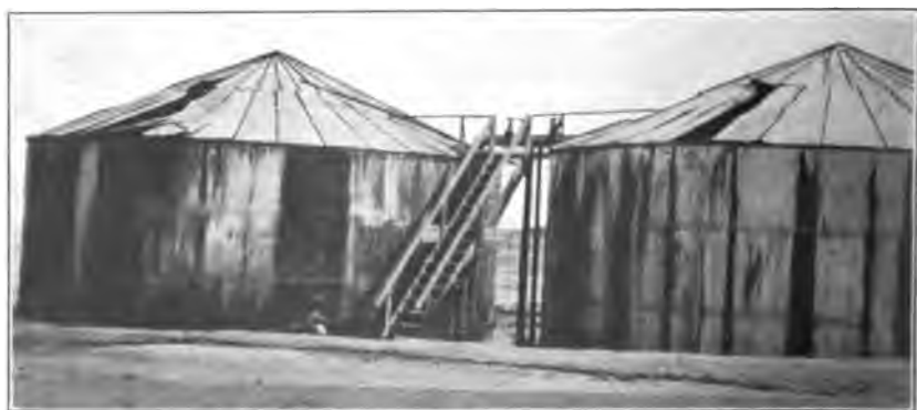
B, LARGE STEEL TANKS WITH BAD ROOF SHOWING NEGLECT OF EVAPORATION LOSSES.
