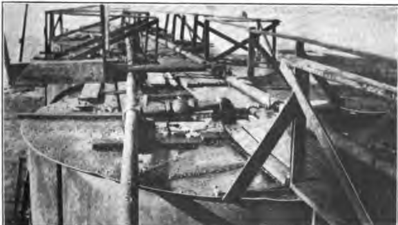
C. TYPICAL CONDITION OF THE ROOFS OF SUCH TANKS AS ARE SHOWN IN PLATE V, B.
