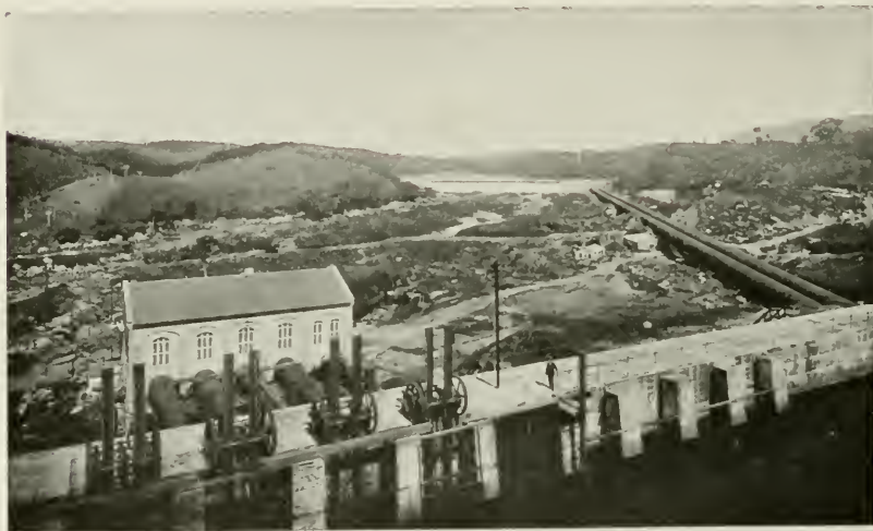
POWER AND LIGHTING PLANT OF SÃO PAULO, BRAZIL.
