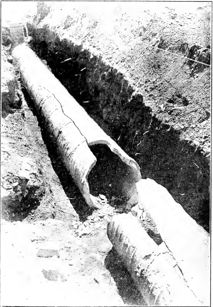
Fig. 5.—Longitudinal crack in 20-inch pipe line. The open section has been broken out with hammer. Photo by W. C. Axelton.
