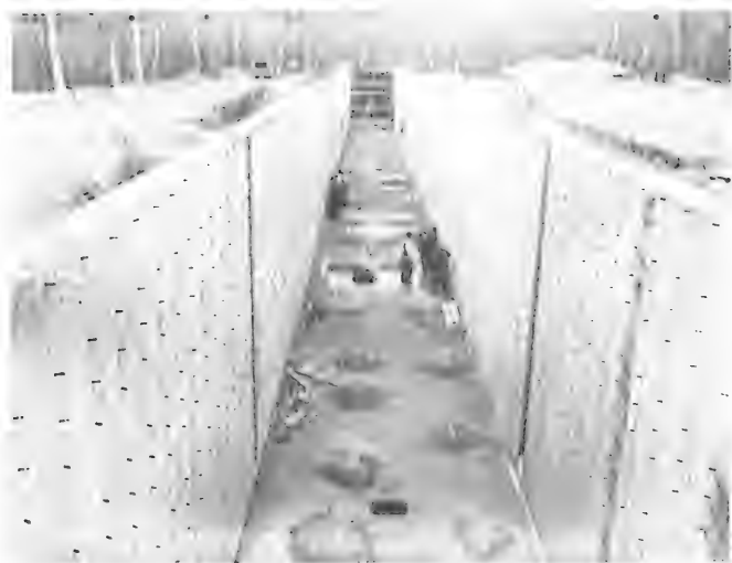
FIGURE 2. WAVE TANK INTERIOR AND CONSTRUCTION OF WAVE GENERATOR SUPPORTING STRUCTURE IN THE BACKGROUND
