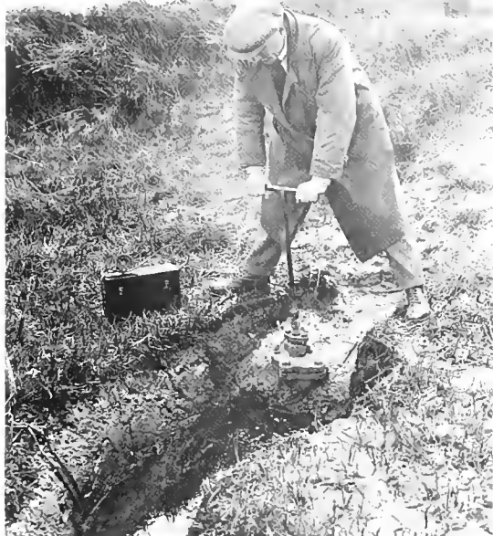
Fig. 20 Draining a salt-marsh area by opening a sluice valve during low tide
