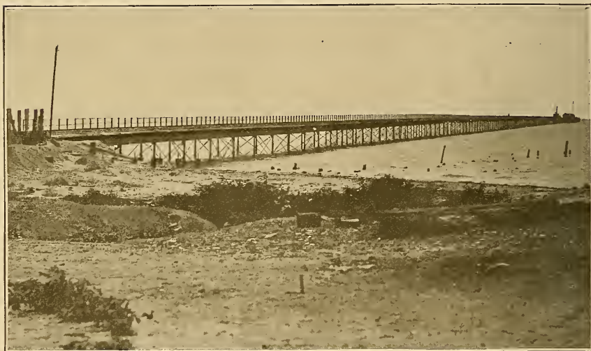
STEEL PILE PIER OF THE BARRANQUILLA RAILWAY AND PIER COMPANY (LIMITED), AT PUERTO COLOMBIA, THE ACTUAL SEAPORT FOR BARRANQUILLA, COLOMBIA.
