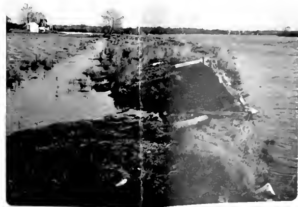
A breached dike at Burcham's farm.
