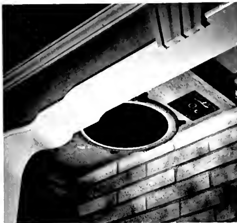
Speaker systems were placed face-down in fireplace casements of the Assembly Room.
