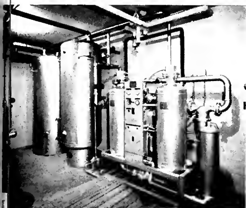
Atlantic Research air dryer equipment takes a moisture out of compressed air before it is supplied to the printing machines on floor above.
