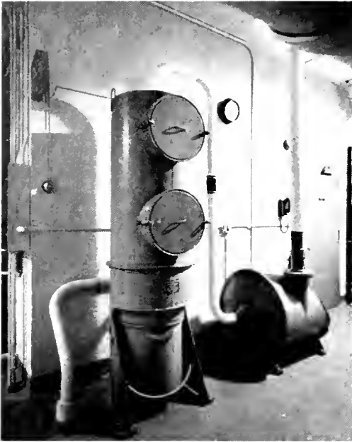
Heart of the vacuum system which keeps entire lab dust-free is this Spencer Turbine machine.
