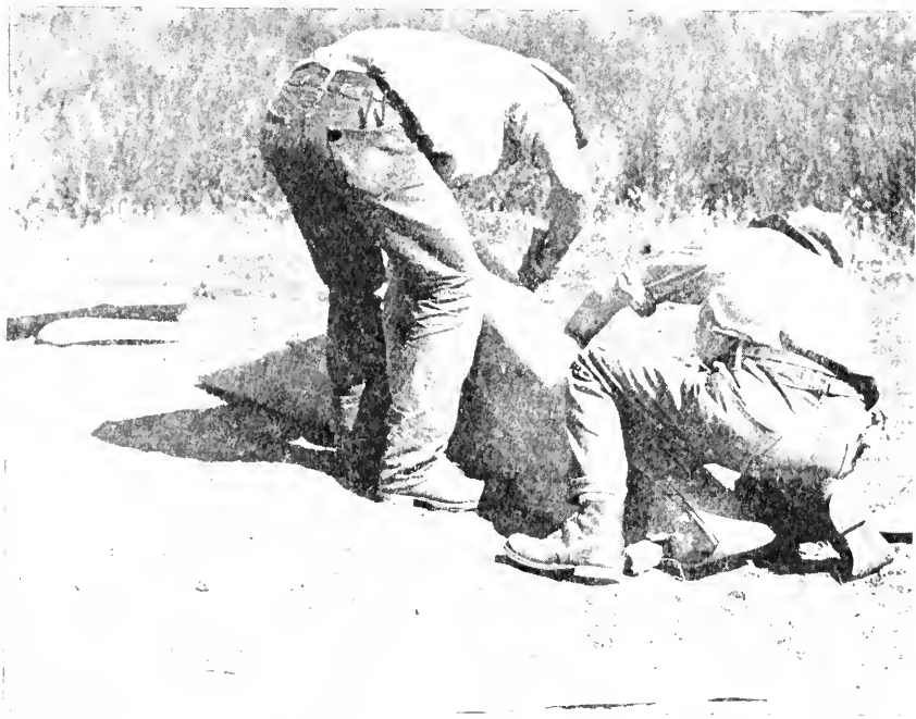
FIG. 48. Covering inside form of trough with building paper to facilitate removal. Note 2-inch pipe attached to lower side of form; this will form the connection between tank and trough.
