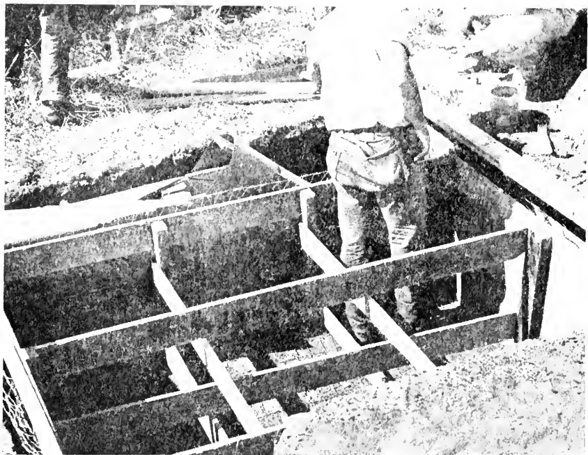
FIG. 49. Tank and trough form in place. Note hog-wire reinforcing between forms and in bottom of tank.
