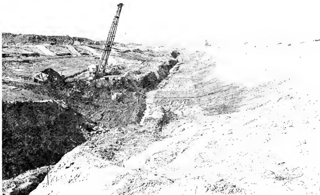
FIGURE 72. Excavation of Delta-Mendota intake canal in progress, July 8, 1948. This view was taken looking toward the site of the pumping plant from the Byron-Bethany Highway
