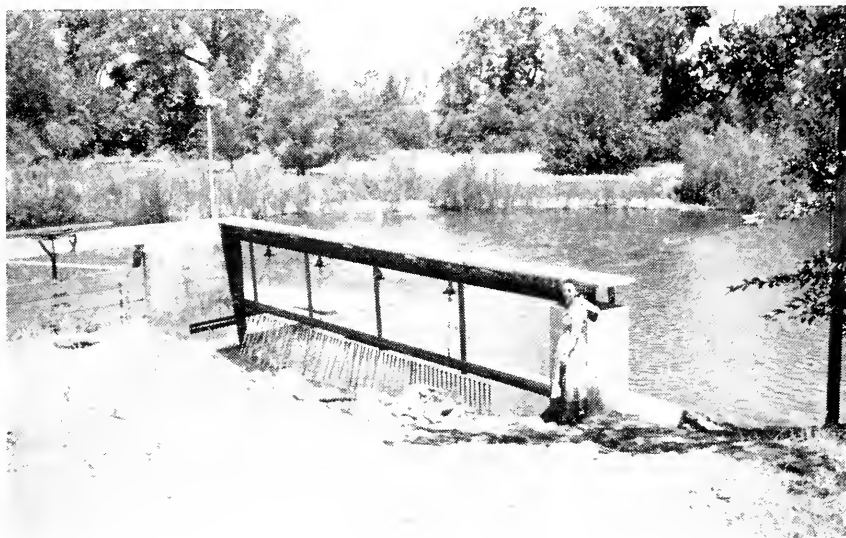
FIGURE 9. Mill Creek electric fish screen
