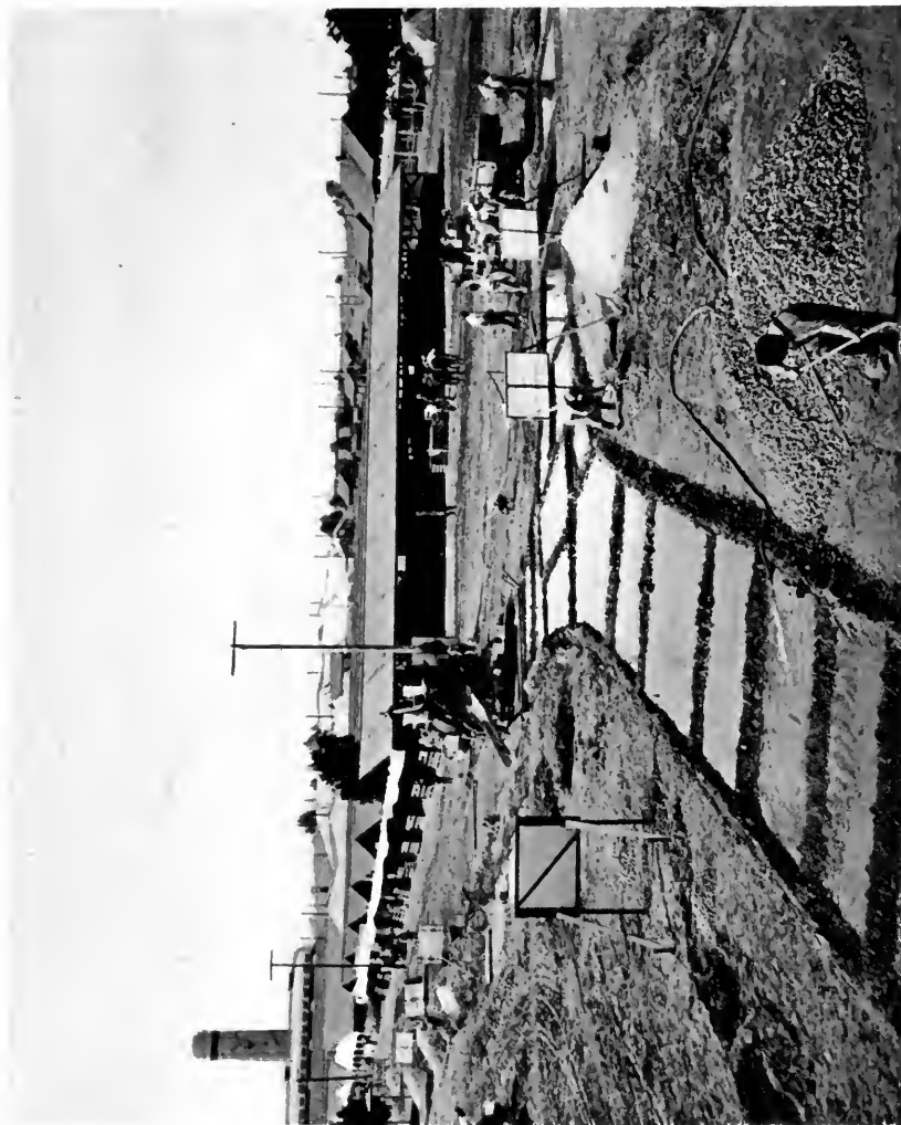
Demonstration concrete highway put down during State Fair at Sacramento. This educational work was carried on during the 1916 State Fair by the California Highway Commission co-operating with the Sacramento County Good Roads Association to boost the County bond issue.
