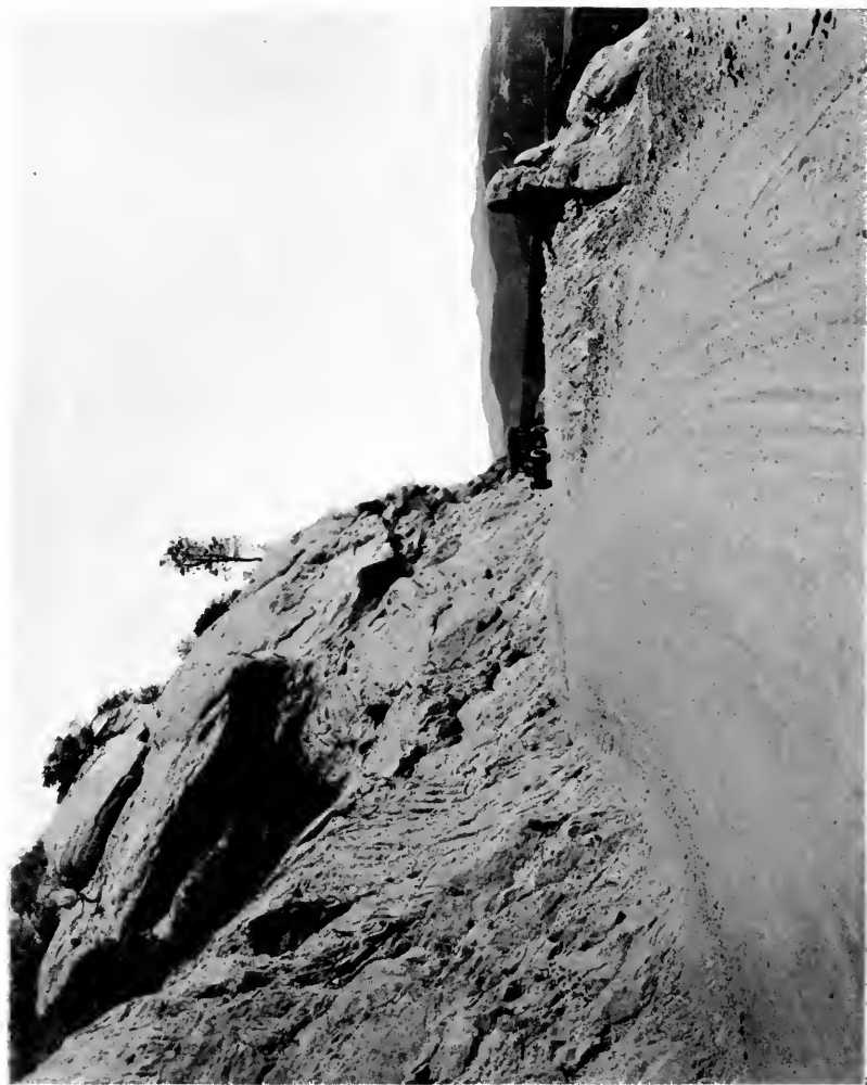
Wide roadways in the mountains form part of the "safety" plans of the California Highway Commission.
