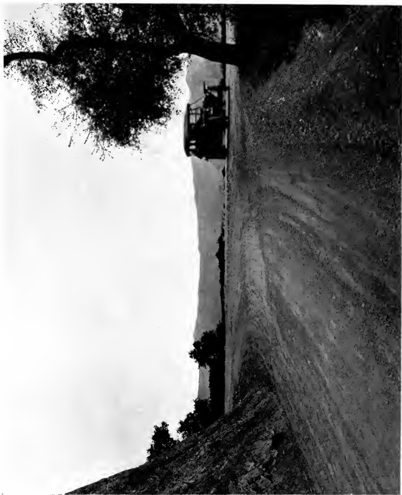
Inspiration Point on the Santa Cruz Lateral of the State Highway. To be paved with concrete.
