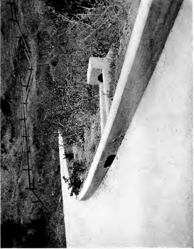
This picture shows in detail the poured curbs used in State Highway work. Corrugated pipe spillway carries off water, preventing bank erosion.
