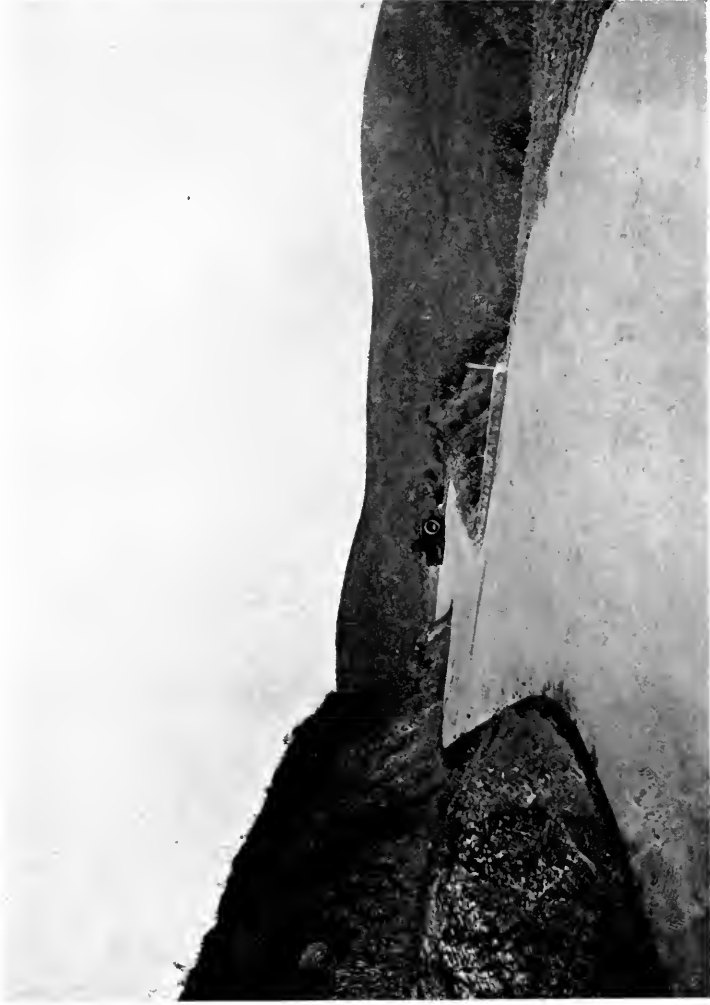
This picture shows in somewhat exaggerated form the super-elevation of curves now supplied in State Highway construction work.
