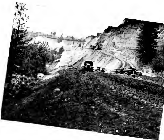
PIONEERING A ROAD along steep cliffs with steam shovel and trucks. Completed embankment is shown in foreground.
