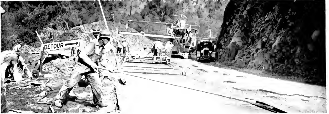
FAST WORK in finishing this new portland cement concrete paving job in Placer County was made possible by several devices created by State Highway engineers.
