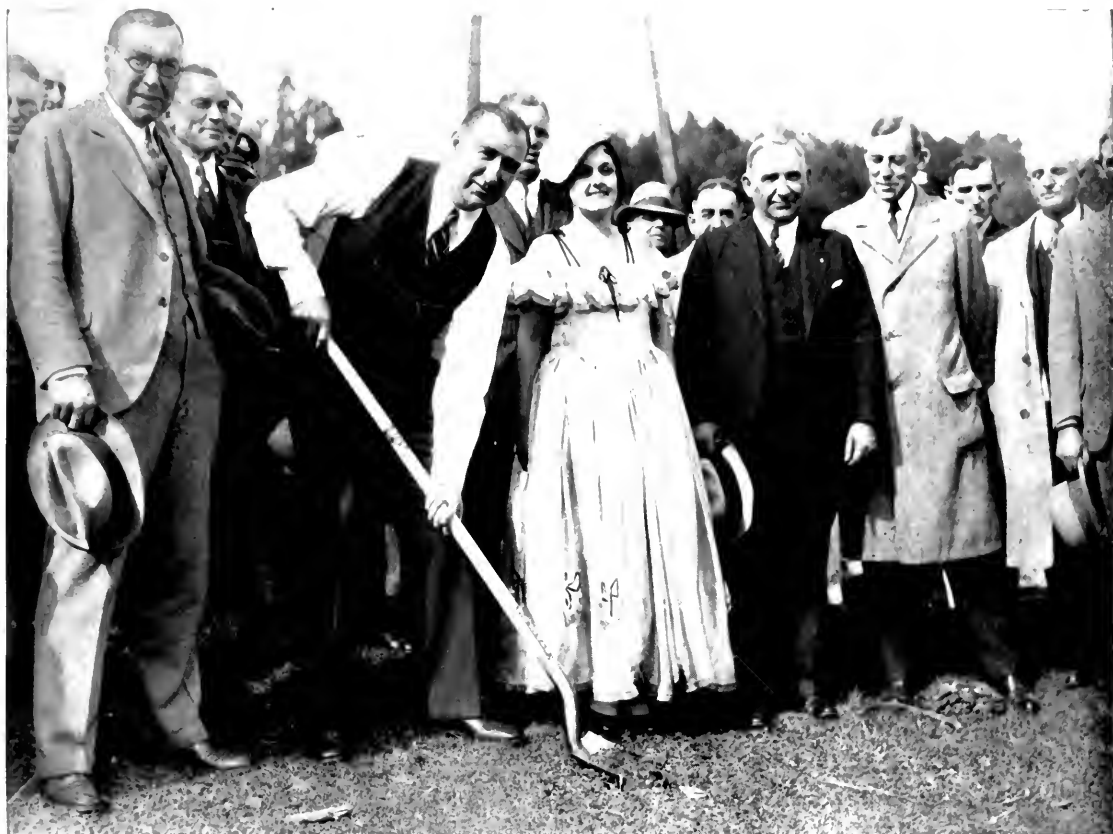
DIGGING IN to start a great highway project Chairman Earl Lee Kelly of the California Highway Commission is shown breaking ground on February 21 for the Cloverdale-Hopland improvement. Left to right, are Senator R. R. Ingels of Mendocino County looking over the shoulder of State Highway Engineer C. H. Purcell; H. G. Ridgway, vice president Redwood Empire Association; Earl Lee Kelly; Harry Lutgens, president Redwood Empire Association; Miss Hazel Hurt, Cloverdale; Colonel Walter E. Garrison, Director, Department of Public Works; Colonel Jno. H. Skeggs, District Engineer; Supervisor Willard Cole, Sonoma; Mayor Charles E. Humbert, Cloverdale.
