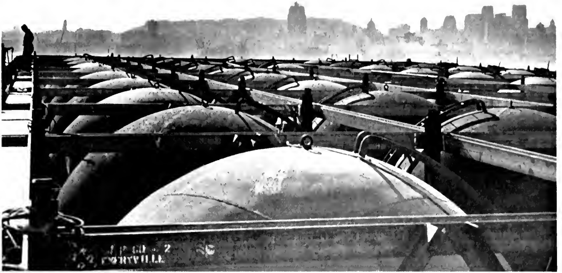
DOMES OF STEEL forming the tops of the 55 cylinders in the world's largest compressed air flotation caisson for the concrete center anchorage of the San Francisco-Oakland Bay Bridge are shown in the above photograph revealing San Francisco's skyline in the background as the caisson is being sunk in mid-bay. The domes are alternately cut off and rewelded into place as the cylinders are increased in height. The caisson is 92 feet wide by 197 feet long and the anchorage when completed will be 478½ feet high and project 298½ feet above water.
