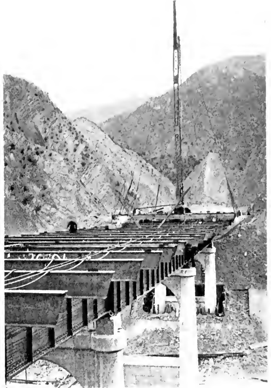
TRAVELING DAYS are nearly over for the steel floor beams being picked up and laid down by a moving derrick on this Piru Gorge bridge.
