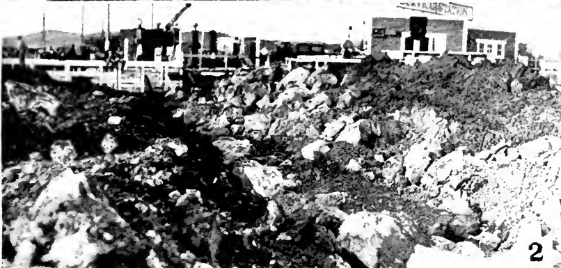
No. 2—This close-up view of the fill started across the tidal flats shown in the above picture illustrates some of the difficulties the engineers are encountering with the 40-foot of mud overlaying the fill foundation. Tons of displaced mud carrying large rocks from the main body of the fill are being forced to the surface.
