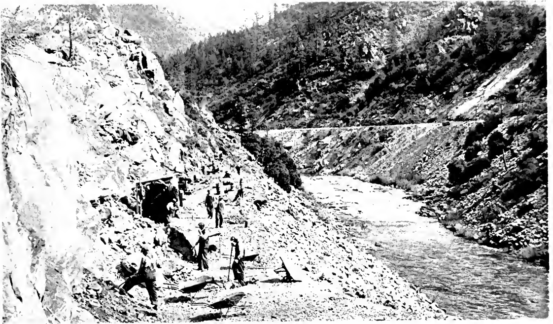
WORKING WITH A WILL for food and lodging, these men of the Rich highway camp for relief of single unemployed itinerants, laboring six hours every working day since December 15, moved 25,000 yards of rock and dirt in widening 1\frac{1}{2} miles of Feather River road trail by handwork.
