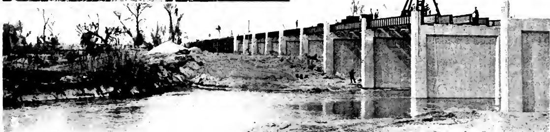
PROFITING BY COOPERATION with the State in rerouting U. S. 99 through the city, Bakersfield will have a fine, wide arterial for through traffic, relieving city congestion and avoiding grade crossings. No. 1—Chester Avenue crossing of Southern Pacific that will be eliminated. No. 2—New bridge over Kern River showing wide concrete deck under construction. Nos. 3 and 4—Views of present narrow old concrete arch bridge at times inadequate for traffic. No. 5—Reinforced concrete piers of new bridge are 54 feet wide.
