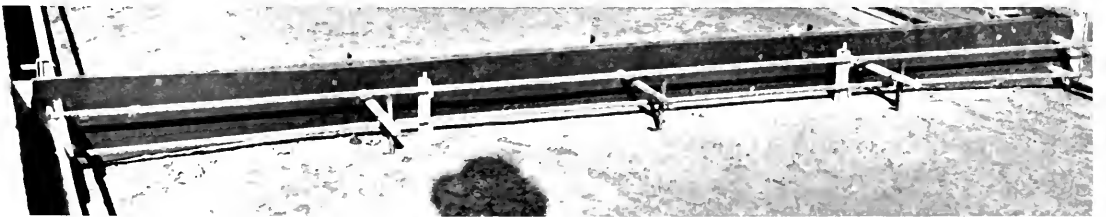
NEW CHAIRS for supporting steel reinforcing bars in expansion joint construction were developed for this paving job in San Joaquin County. The metal chairs are shown supporting the bars.
