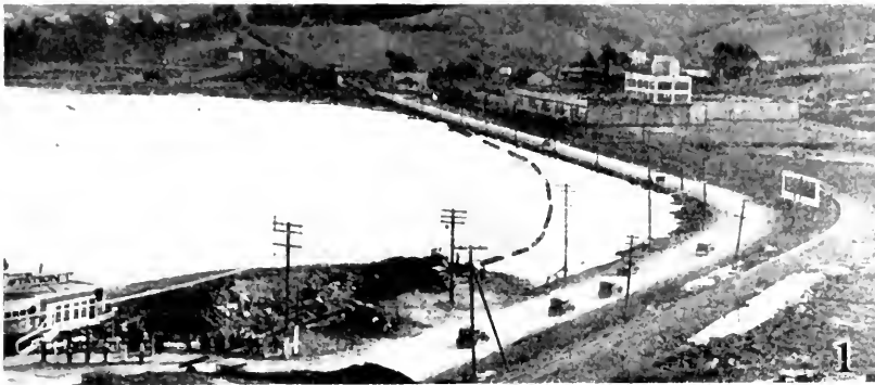
No. 1—Beginning of fill across tidal flats of Richardson Bay near Waldo Point. Dotted line shows approximate new alignment adjacent to present Bolinas Avenue across a natural settling basin where fill must be sunk through 40 feet of mud. New route cuts through hills in background.
