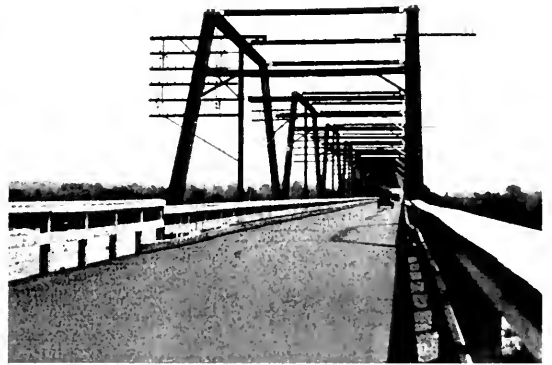
JUNK PILE awaits this narrow old wooden structure with its unsightly overhead girder trusses built in 1898.
