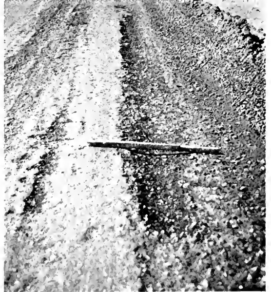
NOT ENOUGH OIL in the mixture produces a surface that becomes badly raveled under traffic.
