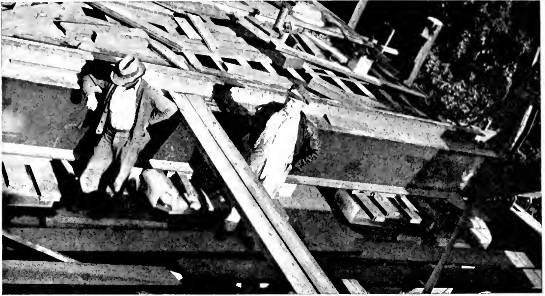
A MELTING SCENE —Here's the iceman helping the engineer watch six cakes of ice do the work of jacks in lowering bridge truss.
